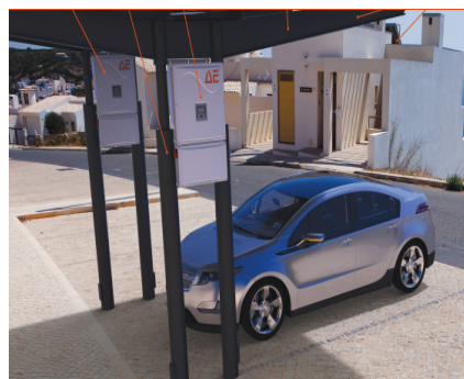
Figure 6: AE 3TL 17(867) 17KW grid tied Inverter
